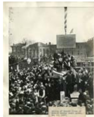
Laying of the courthouse cornerstone. Photo courtesy of the Monroe County History Center
