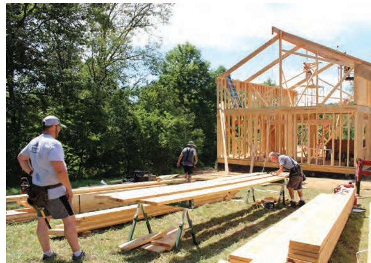
(l-r) Dylan Grigar, Scott Rodriguez, and Rick Dyer on a build site. Courtesy photo
